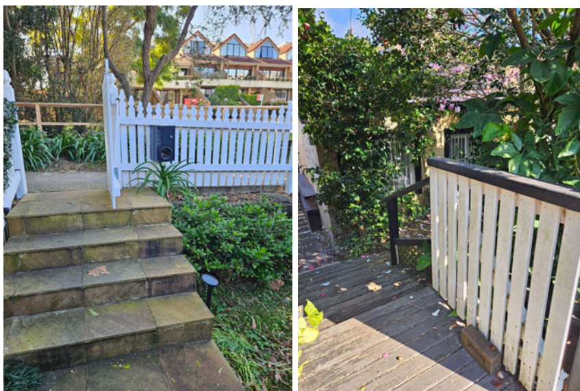
Images 3 & 4: Steps from footpath to get down to front door below footpath level.
