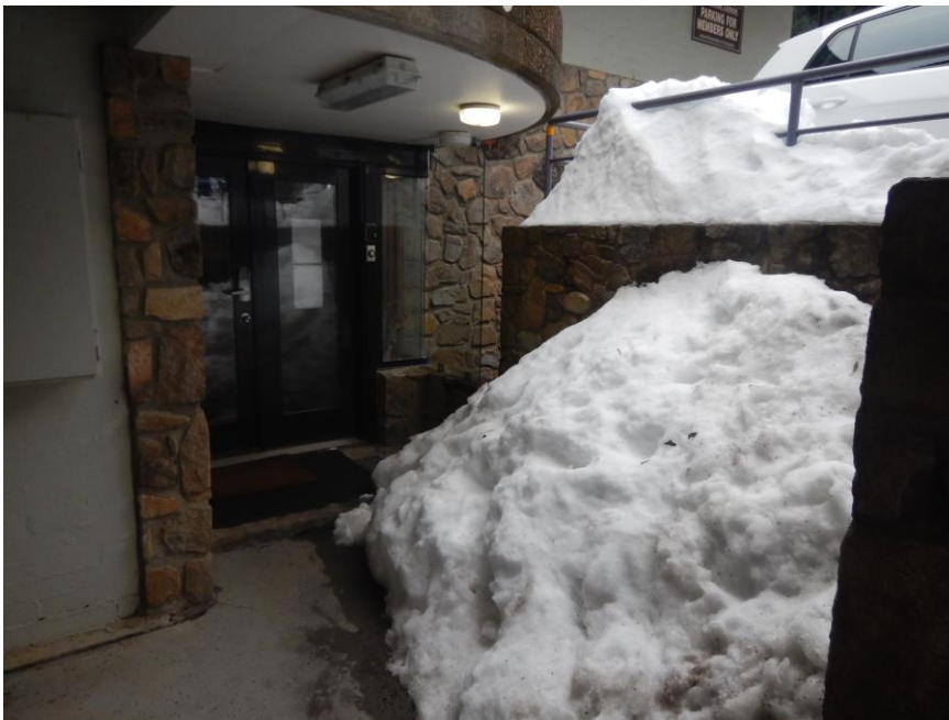
Figure 13: Snow deposition within the main entrance
