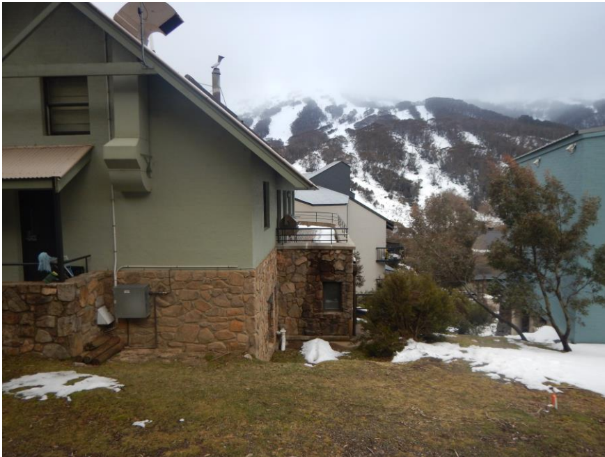
Figure 8: Current roof line sheds snow directly onto the deck with no snow barriers
