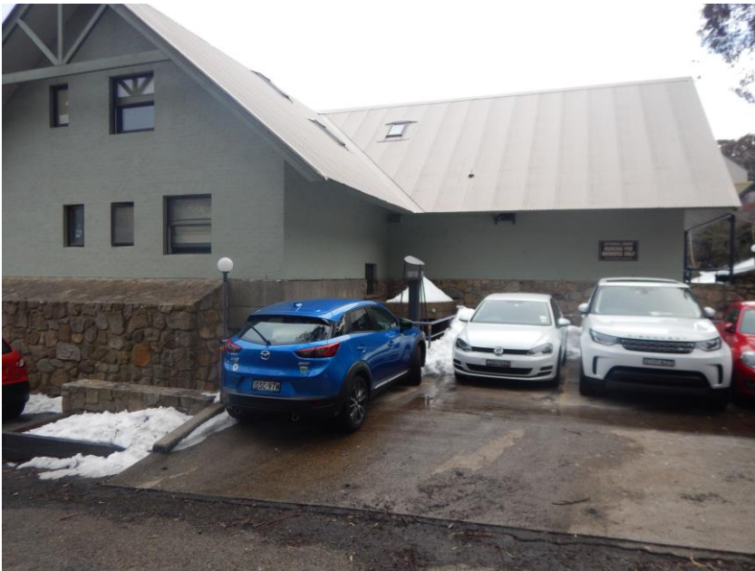
Figure 11: Both roof planes and valley concentrate snow deposition over the main entrance
