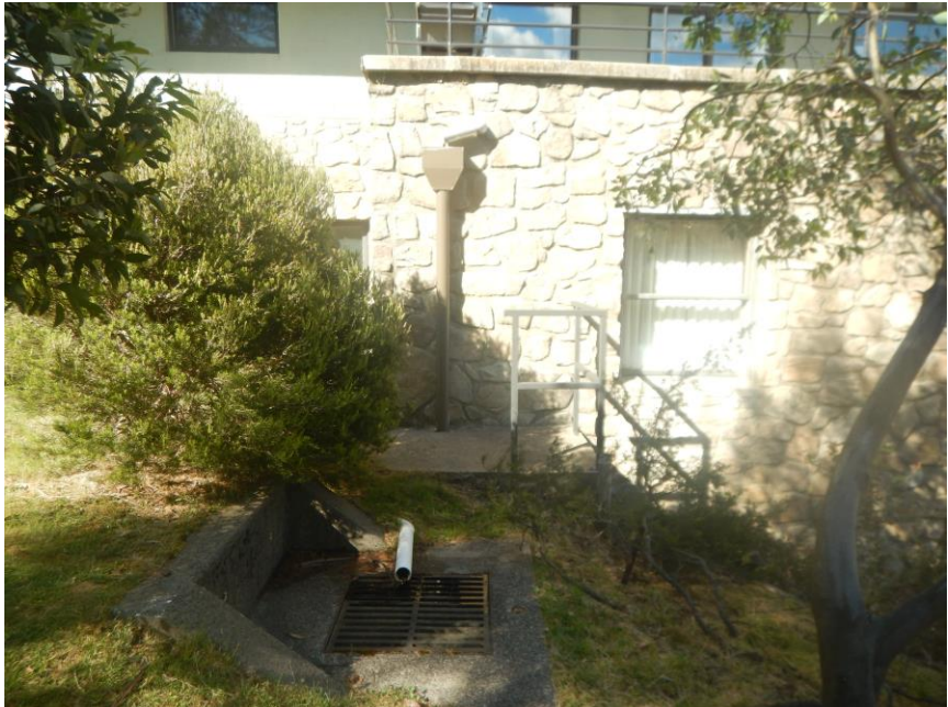
Figure 8: Photo of the existing stormwater below the proposed extended deck and roof
