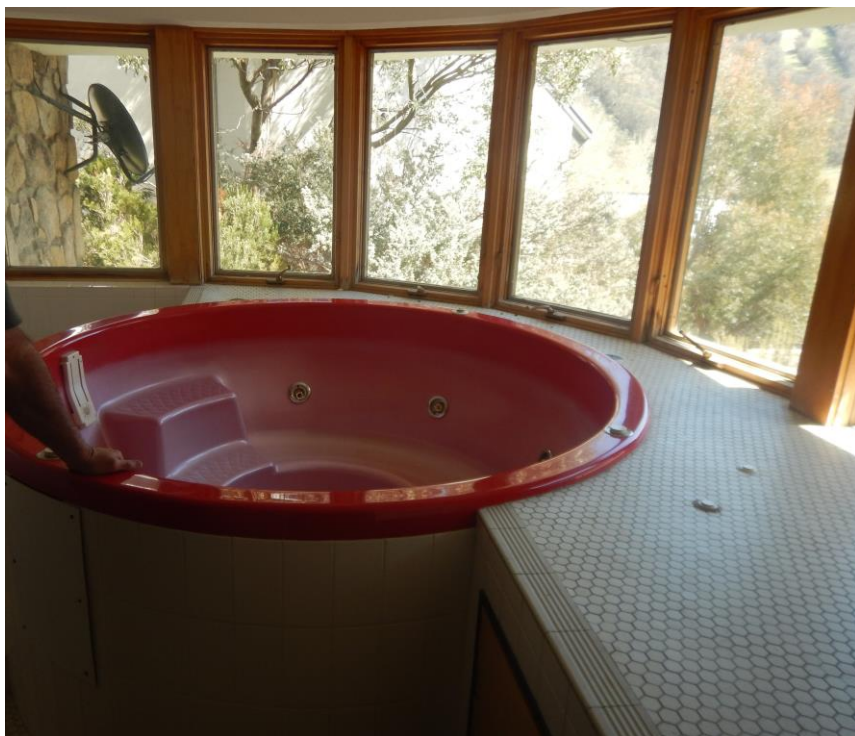
Figure 14: Existing spa to be removed and room to be used as a small lounge area
