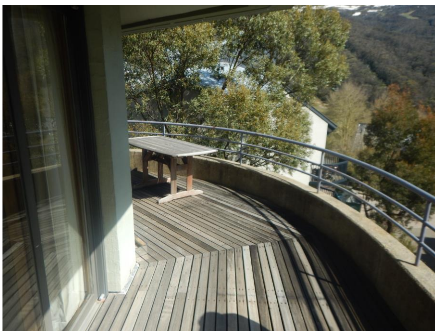
Figure 7: Current deck is not deep enough, subject to snow deposition with a non-compliant balustrade
