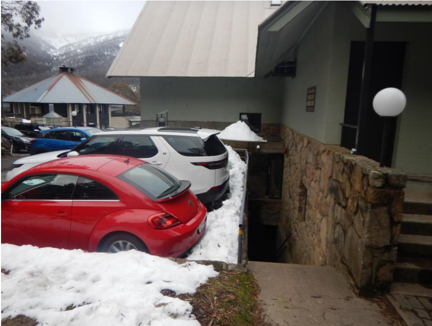
Figure 10: Car park at the southern side of the building is subject to snow deposition from the roof above
