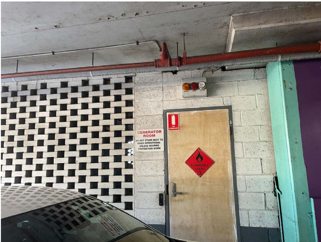
Photograph 12 Generator room with flammable liquid storage.
