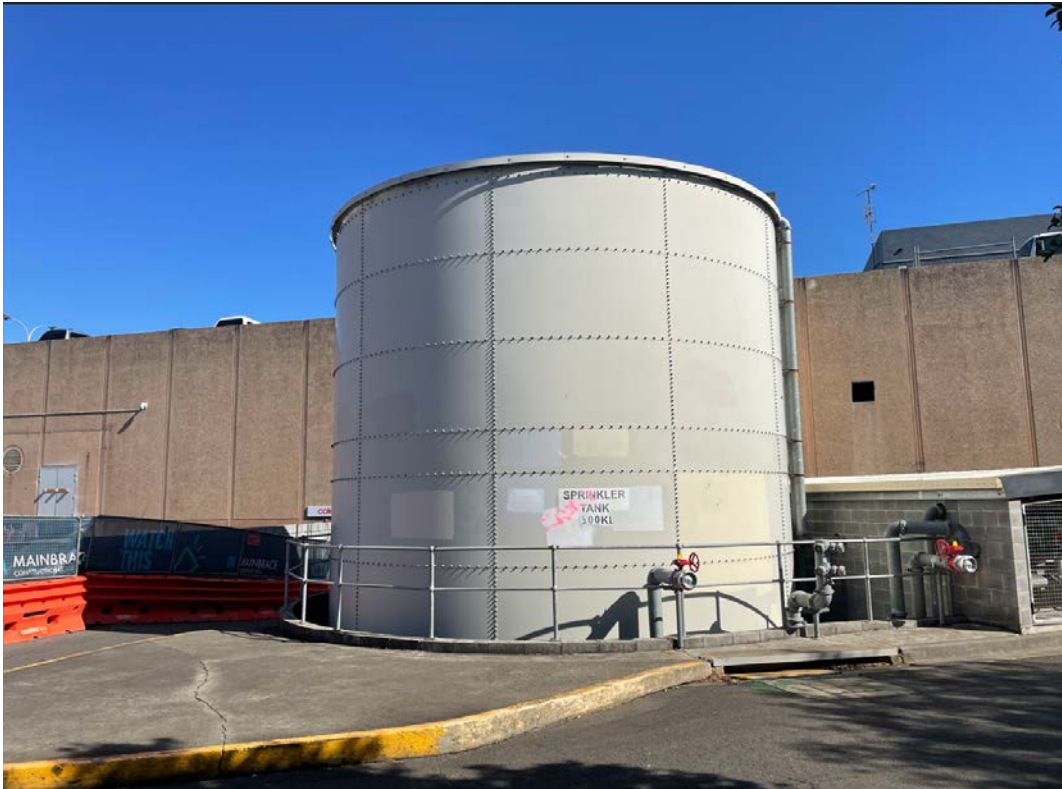
Photograph 17 A large water tank noted on the eastern boundary, used for storage of water for the site's sprinkler system. .
