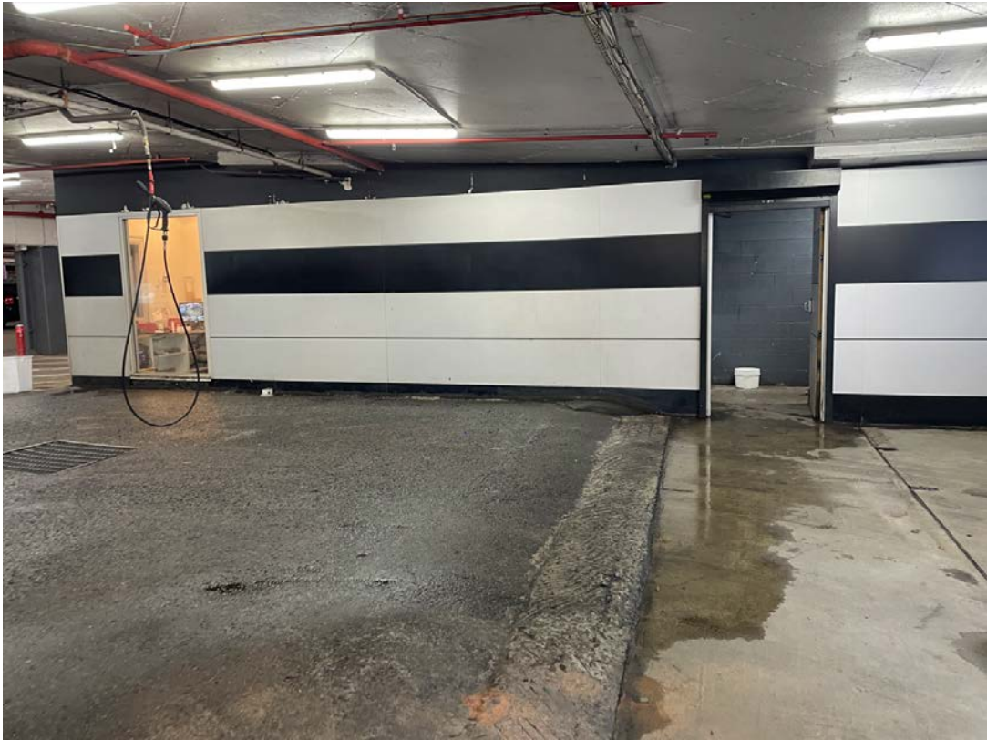
Photograph 13 Car-wash facility located in the ground-floor car parking area.
