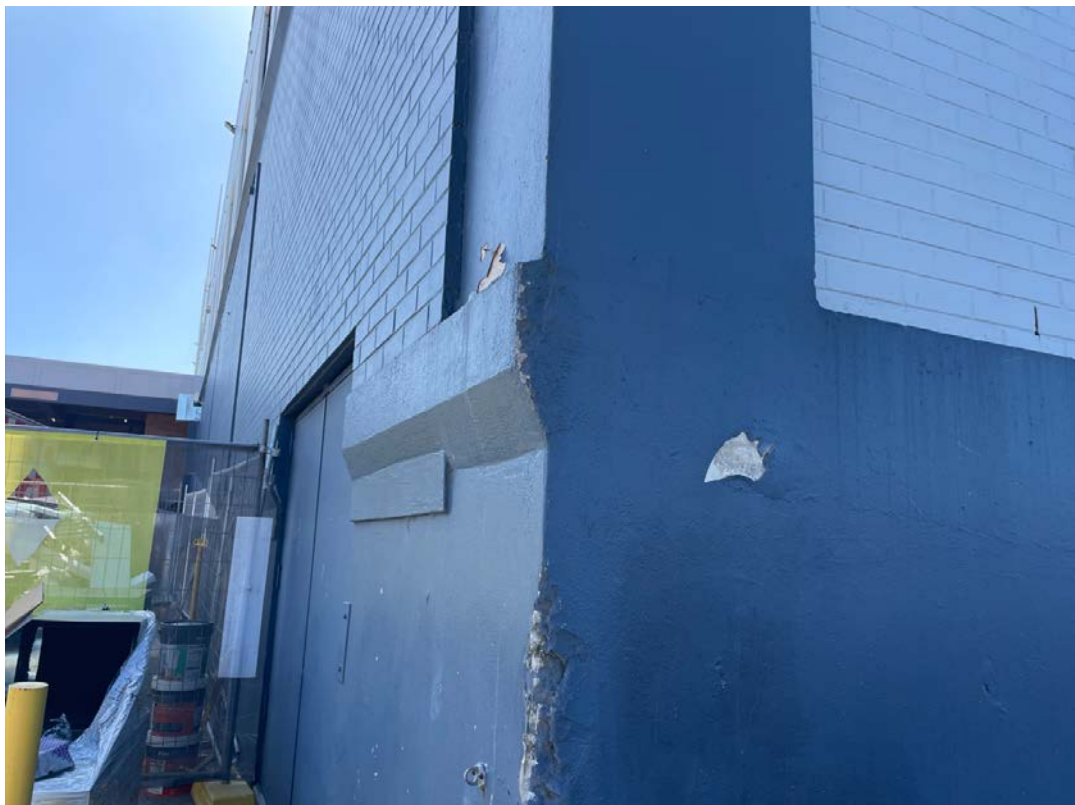
Photograph 2 Building fabrics with paint peeling on the exterior walls.
