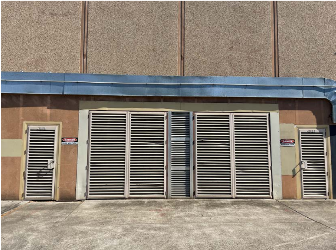
Photograph 11 Electrical sub-station located in the eastern portion of the site.
