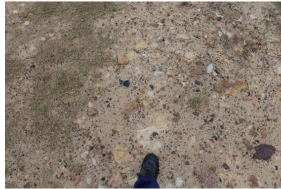
Plate 14. Detail of exotic sandstone rubble used as top dressing for road, excavated to approximately 1.25 metres depth.
