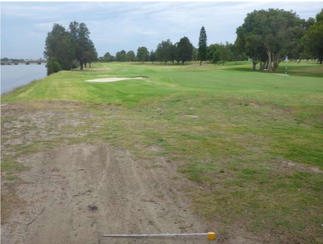
Plate 9 Exposure associated with small scour adjacent to Cooks River, view south.
