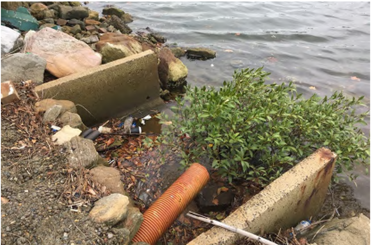
Figure 23: Degraded outfall to the Cooks River at Kogarah Golf Club (photograph taken on 17/03/2017)
