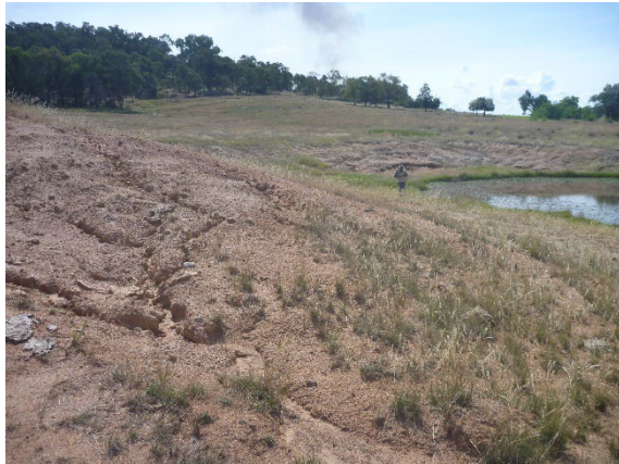
Photograph 8.3: Evidence of earth movement associated with dam features (ERM 2022)
