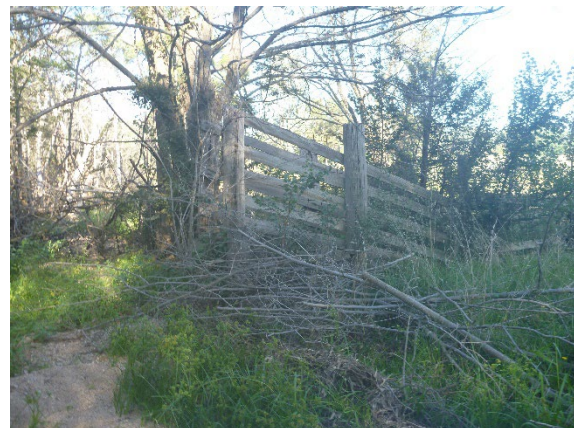
Photograph 10.13: Timber ramp on boundary of property
