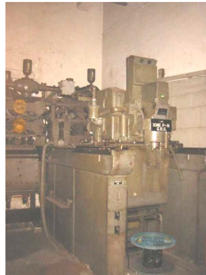
Bus Bar Circuit Breaker
