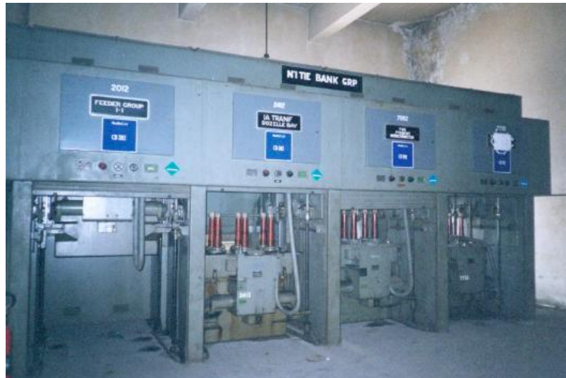
No. 1 Tie Bank Group
