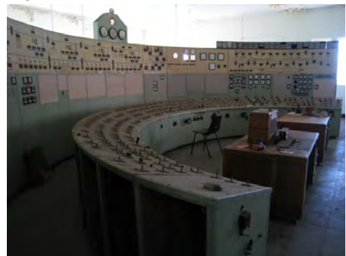
Figure 2.1.2.6 Interior of the Control Room
