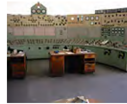
Control Room – total environment
