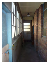
1948 Switch House corridor top level
