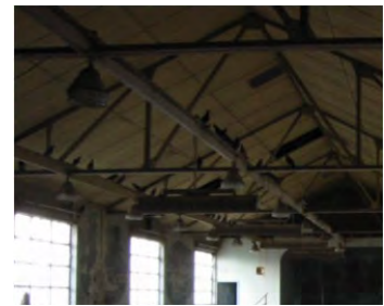
Figure 5.3.8.1 Roosting inside entertainment room, top level of Switch House.
