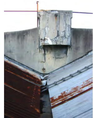
Figure 5.3.2.1 Failed Water Tank (Design 5 - Architects)
