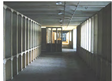
Figure 3.2.2.8 Switch House (Design 5 - Architects)
