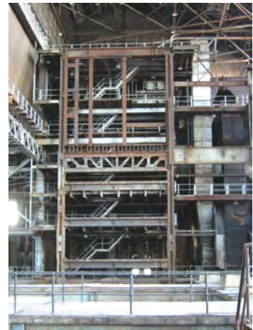
Figure 5.1.7.2 Existing Boiler (Design 5 - Architects)
