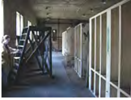
1948 Switch House top level
