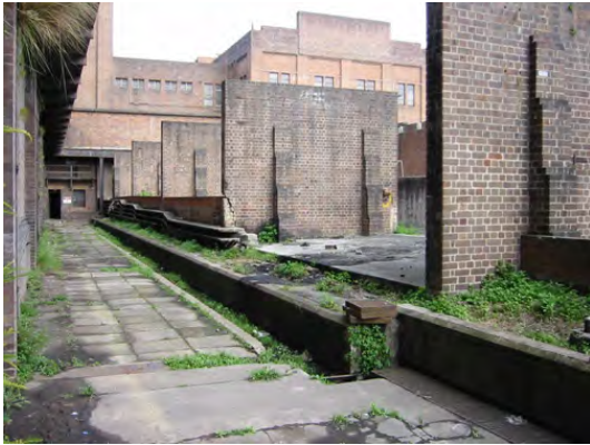
Figure 2.1.1.12 North Transformer Yard (Design 5 - Architects)
