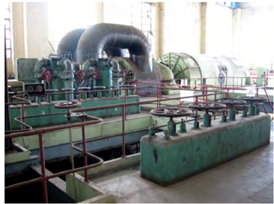
Figure 2.1.1.7 Turbine Generator in Turbine Hall (Design 5 - Architects)
