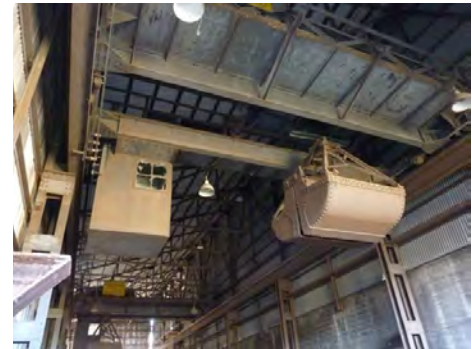
Figure 5.1.5.1 Coal Handling Shed Machinery (Design 5 - Architects)
