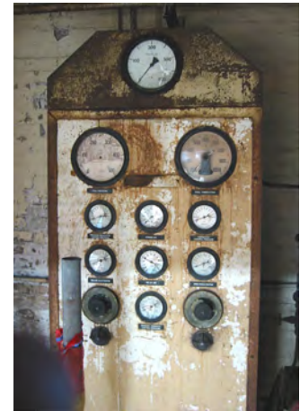
Figure 5.1.3.2 Coal Handling Shed Equipment (Design 5 - Architects)
