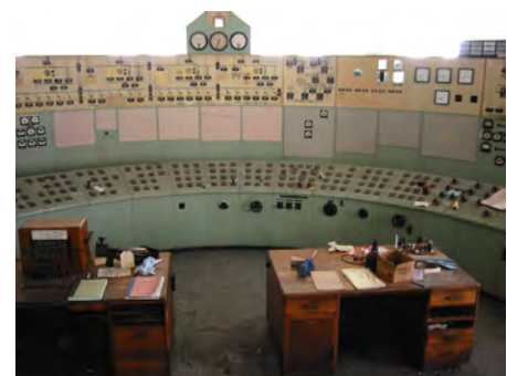
Figure 3.2.2.7 1948 Control Room (Design 5 - Architects)
