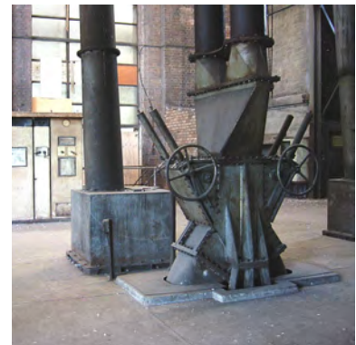
Figure 5.1.1.1 Boiler House machinery (Design 5 - Architects)
