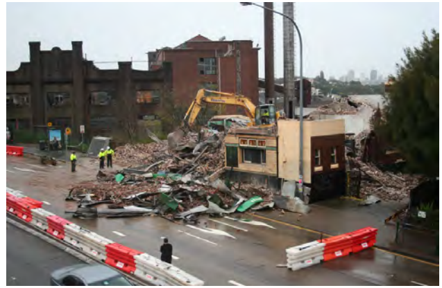
Figure 2.6.9.6 White Bay Hotel demolition, 6 September 2008 (Source: Peter Fletcher Available through Wikimedia Commons, file: White Bay Hotel.jpg)
