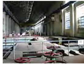
Turbine Hall – space and machinery
