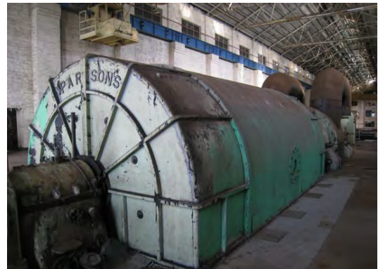
Figure 5.1.8.5 Turbine Hall Machinery (Design 5 - Architects)
