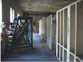
1948 Switch House top level
