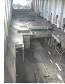
Turbine Hall – platform areas where turbine generators have been removed
