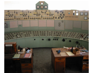
Control Room (Design 5 - Architects)
