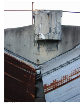
Failed water tank over Admin. section (Design 5 - Architects)
