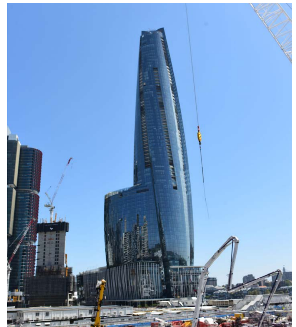
Figure 174 The Crown Sydney Hotel Resort (Block Y) under construction (Source: AECOM, May 2020)
