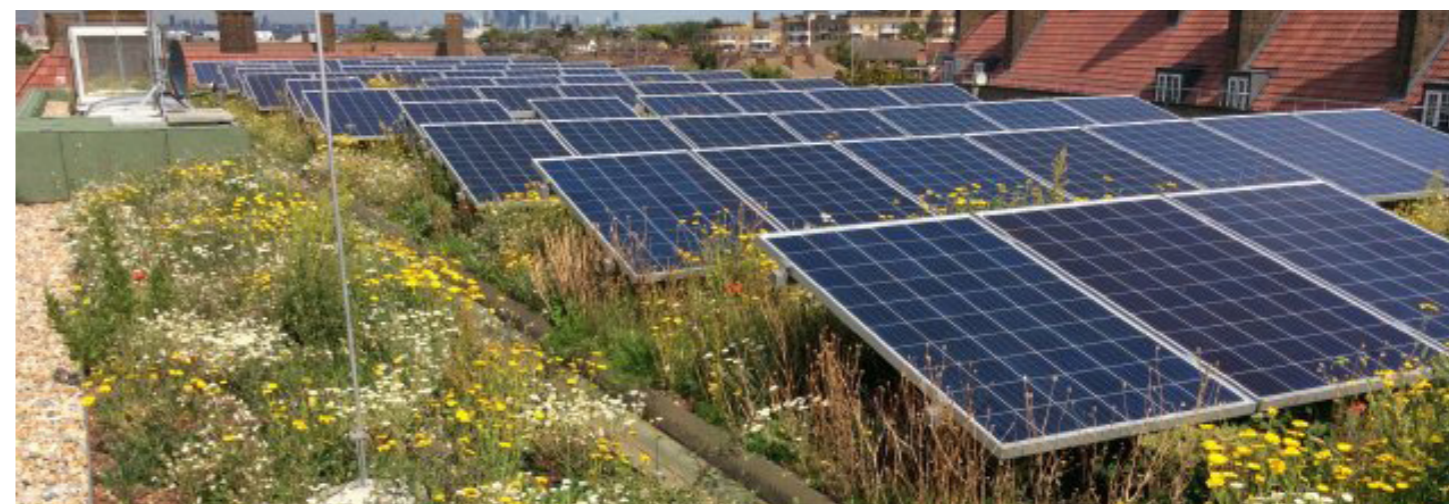
Figure 2.4 Biosolar roof combining solar panels with green roof (Source: Living Roofs)
