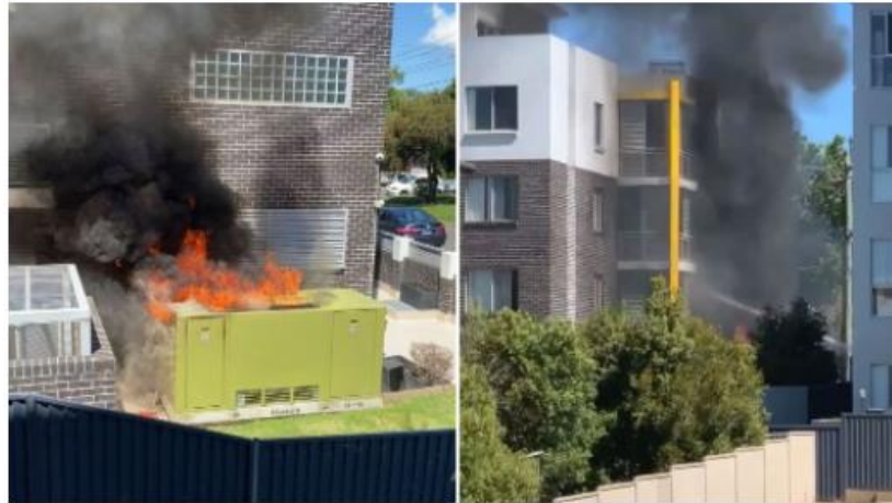
An electrical transformer caught alight in Sydney's south-west today. (9News)
