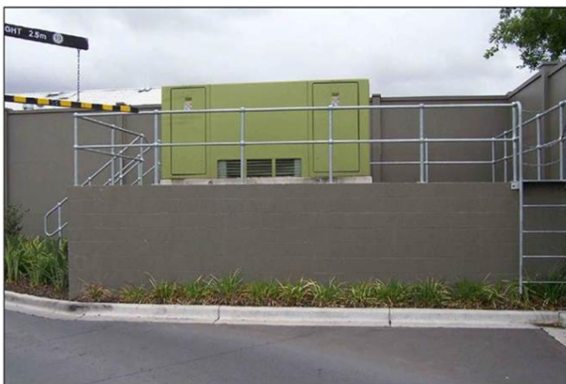
Figure 51 - Example substation raised above 1:100 flood level
