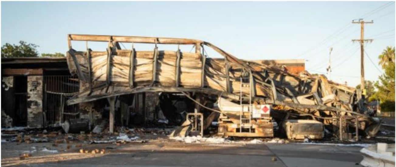
Figure 4: Service Station Facility Following Fire
