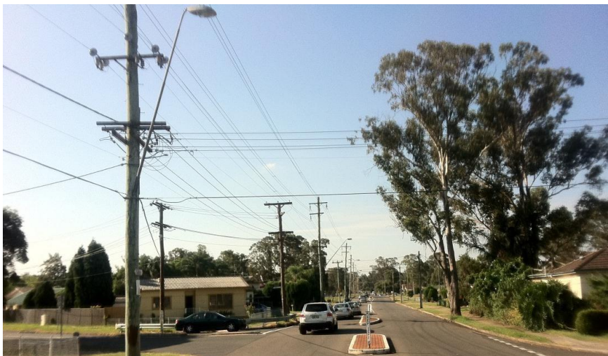
Overhead powerlines with high voltage, low voltage and service connections at different levels on the poles. This example is in Marayong NSW part of Endeavour Energy's franchise / network area. Source: Google Maps Street View.
