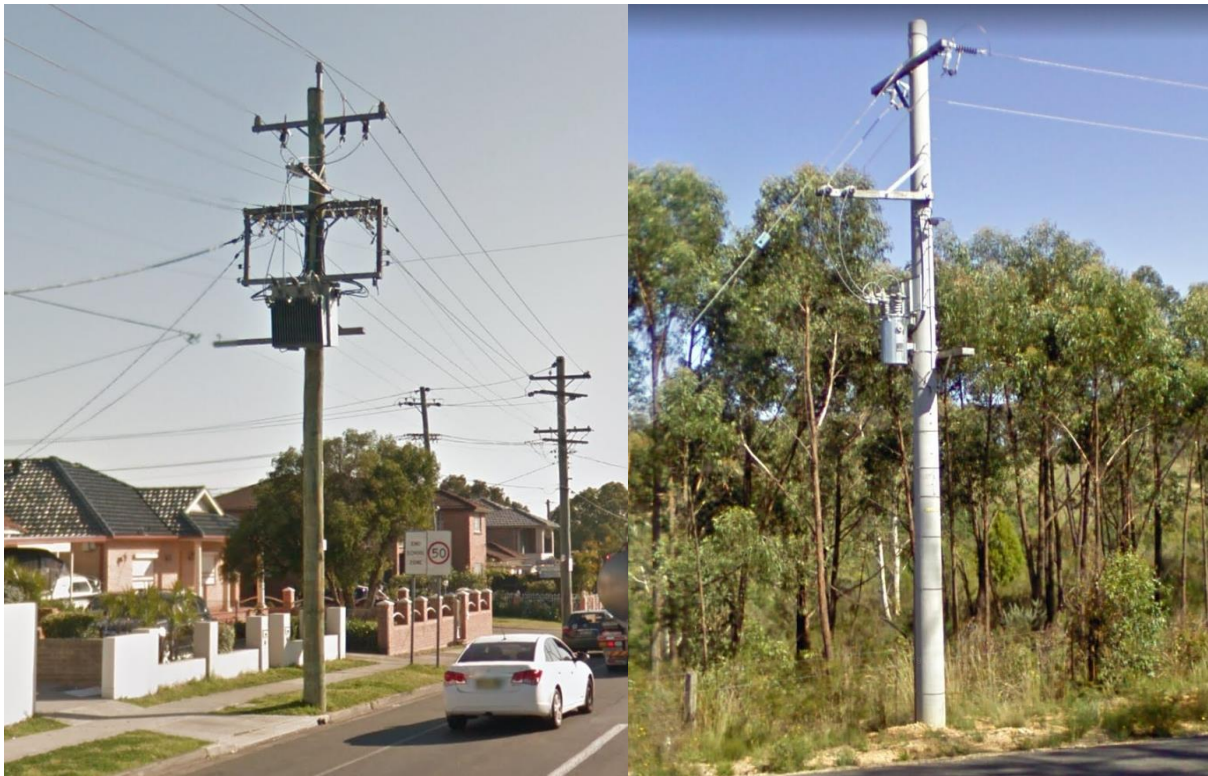
Pole mounted substation no. 914 in Blaxcell Street, Guildford NSW has 79 customer connection points servicing 119 premises in an urban context which is at the upper end of the number of premises able to be serviced. In contrast pole mounted substation no. 26132 in Baaners Lane Little Hartley NSW in a non-urban context only services a single rural property. Source: Google Maps Street View.
