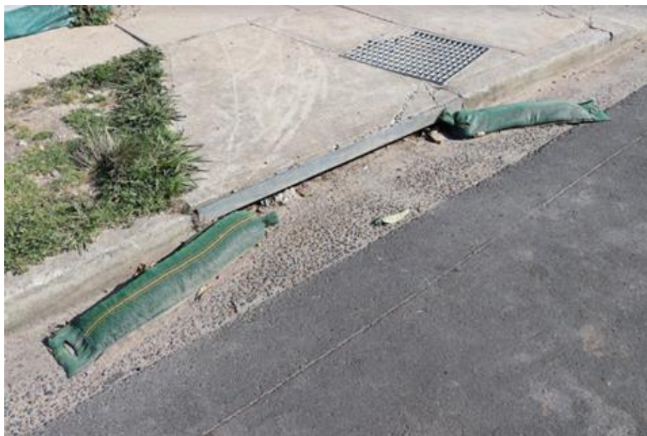
Figure 10. A sandbag kerb sediment trap collects sediment before it can enter the stormwater drain. Source: Parramatta River Catchment Group.
