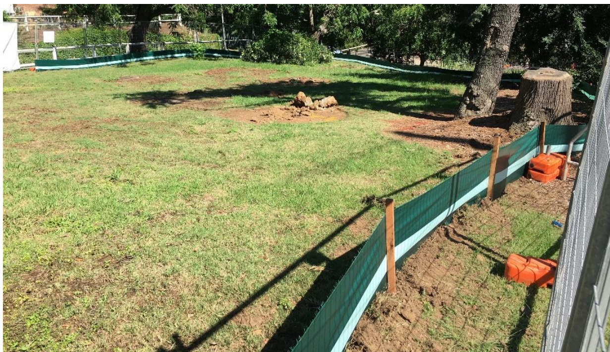
Figure 8. An appropriately installed sediment fence
