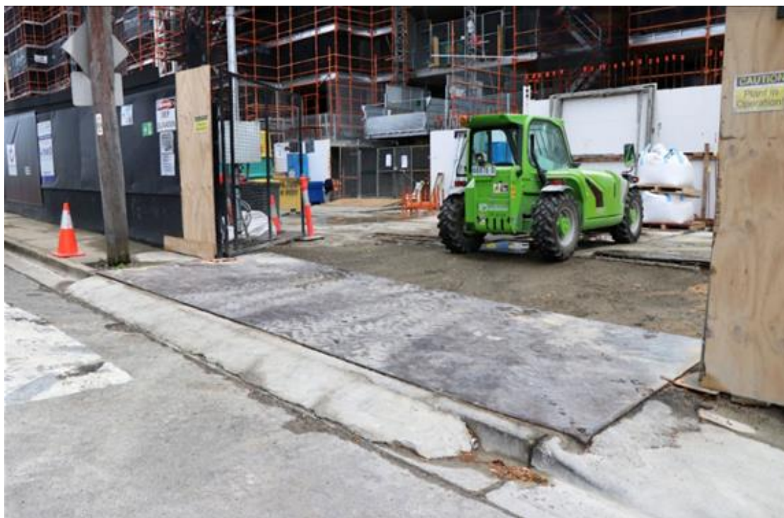
Figure 5. A stabilised site access point. Source: Parramatta River Catchment Group
