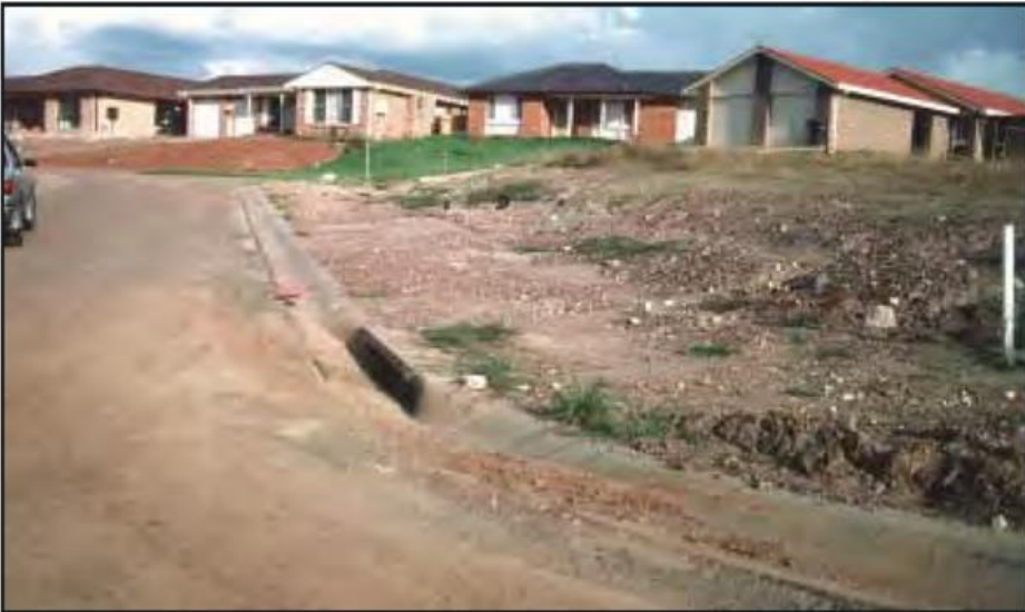
Figure 14. A poorly stabilised site resulting in sediment runoff onto nearby roads and into drains. Source: Managing Urban Stormwater: Soils and Construction , 4th edition.
