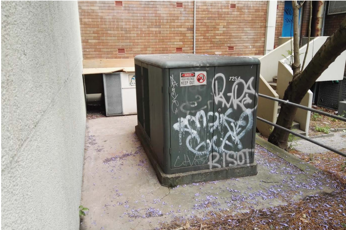
Photograph 9: Substation in the east of the site area
