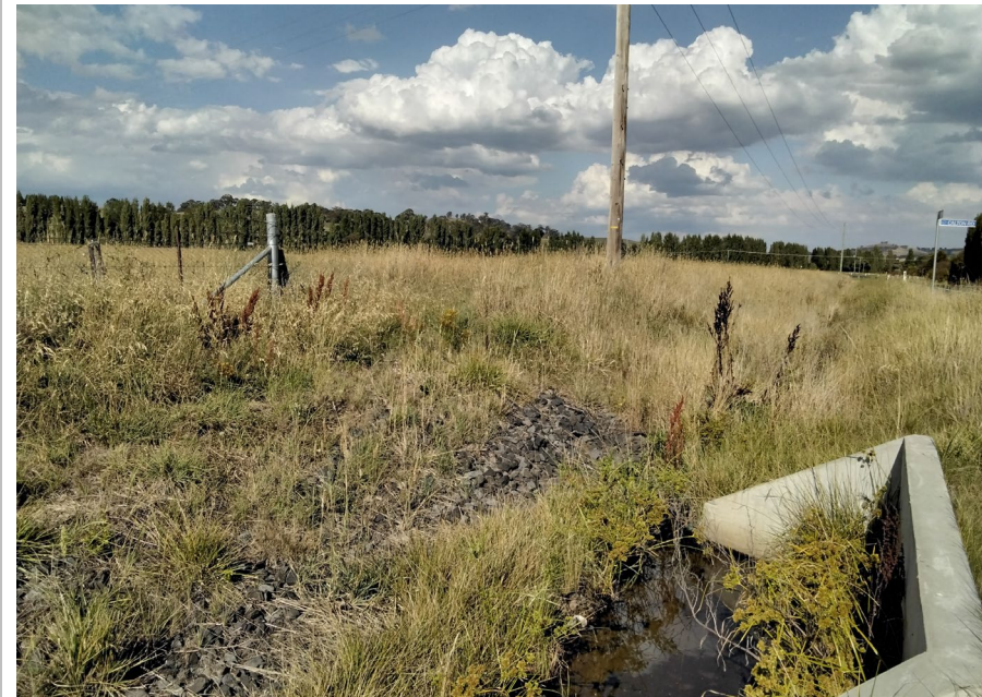
Photo 8 Culvert noted within the southern boundary of Lot 200, adjacent to Dairy Creek Road (photo dated 30/01/2024)
