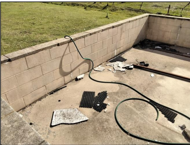
Photo 13 Former AST bund with broken cement sheeting (30 January 2024)
