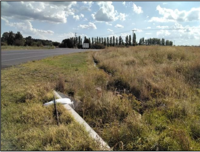
Photo 25 Culvert beneath the Southern Feeder Road within the southeastern corner of Lot 200
