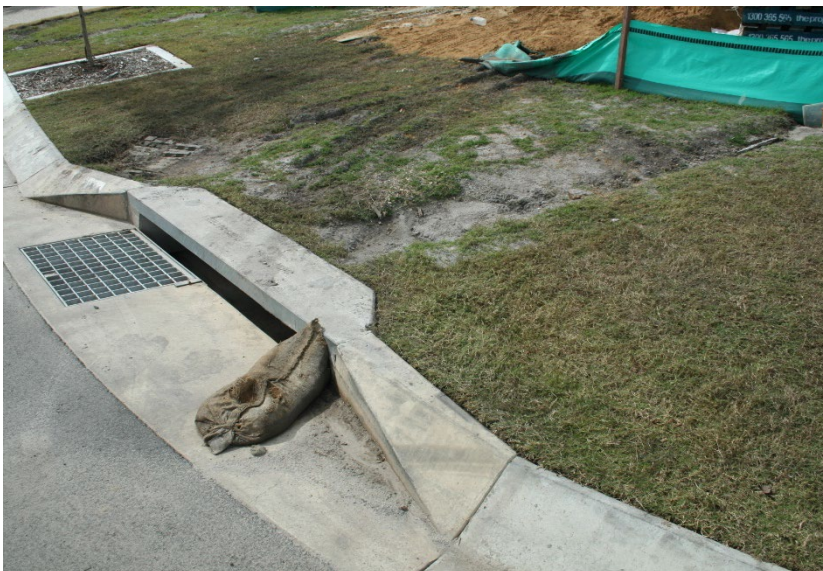
Figure 11. A sandbag kerb sediment trap collects sediment before it can enter the stormwater drain. Source: Catchments and Creeks Pty Ltd
