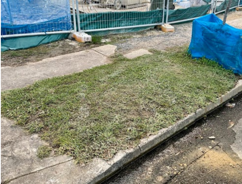
Figure 13. Grass strips by a road that control sediment in low flows. Source: Parramatta River Catchment Group
