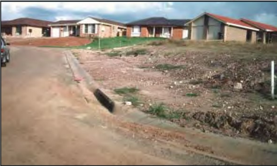
Figure 16. A poorly stabilised site resulting in sediment run-off onto nearby roads and into drains. Source: Managing Urban Stormwater: Soils and Construction , 4 th edition
