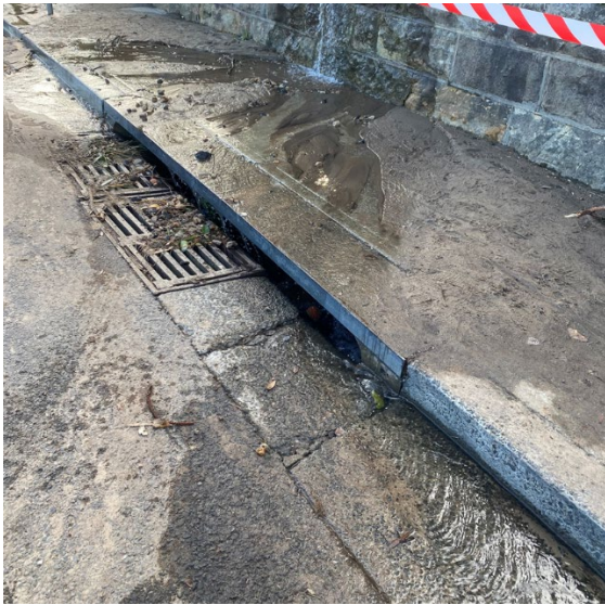
Figure 12. Sediment and debris are affecting a stormwater drain without a sandbag kerb sediment trap
