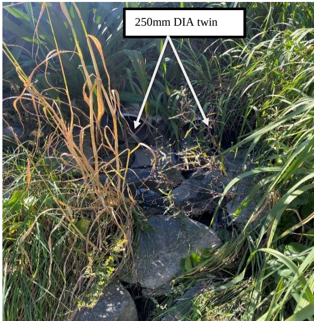
Figure 12: Outlet 3: Twin 250mm diameter stormwater pipe East of Marina Drive
