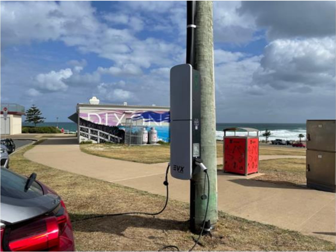
Figure 12 Pole mounted EV charging unit
