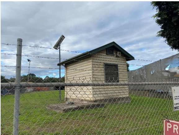
Figure 5 Valve house at 41 Grand Ave
