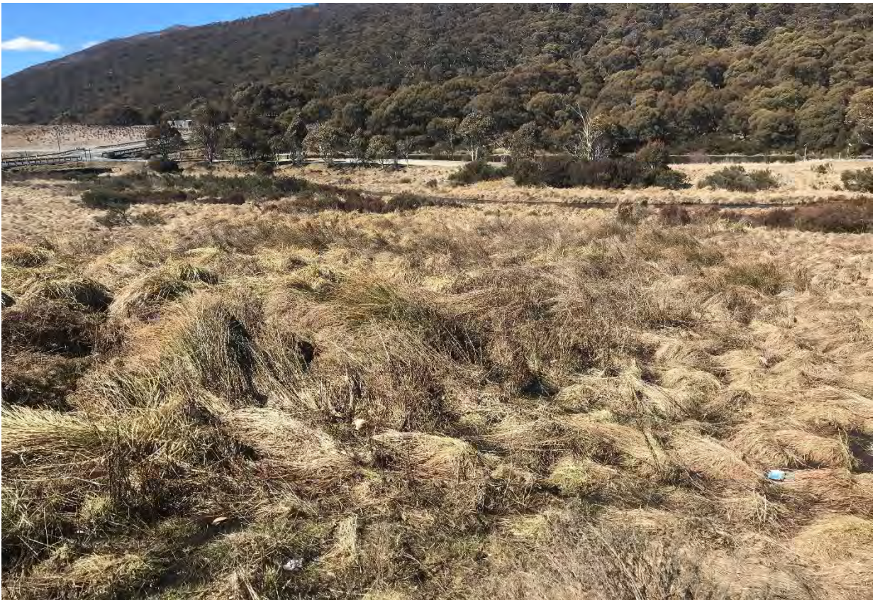
Photo 4: A large culvert discharges water draining off Friday Drive to the central parts of the development site. This has altered the hydrology of this area making it extremely wet and dominated by rushes and exotic grasses.
