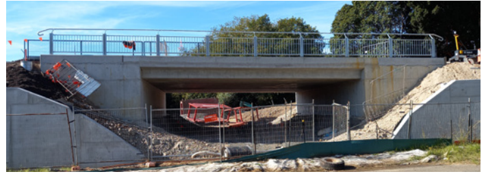
The Parramatta Light Rail viaduct east of the bridge over James Ruse Drive
