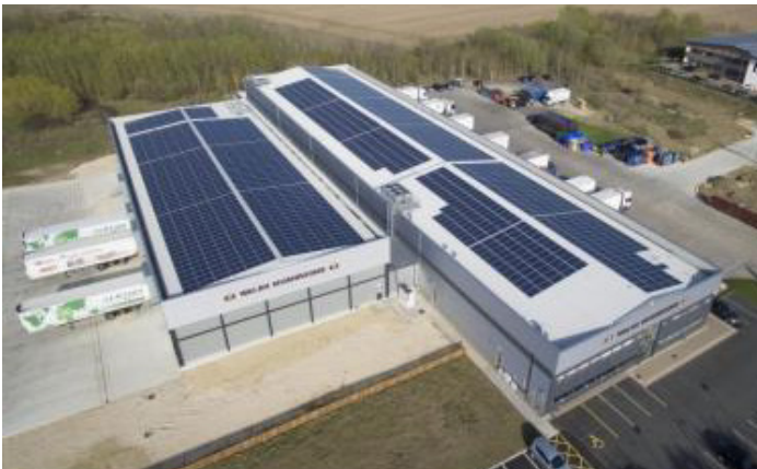
Solar panels on large expanses of industrial building rooftops
