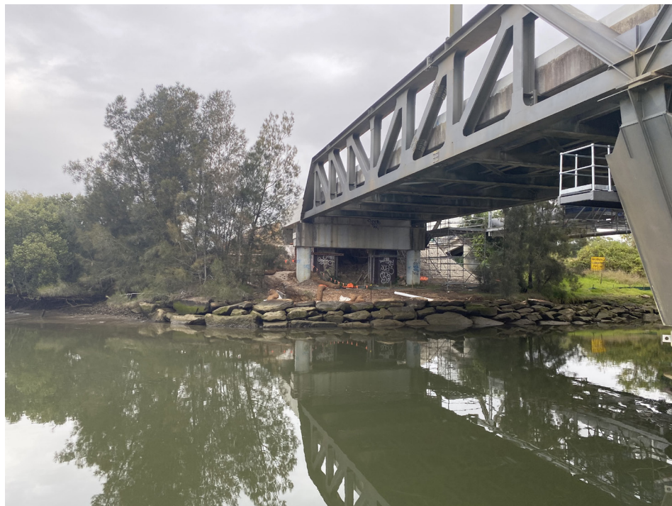
11. The bridge sidings are currently partially buried but should be uncovered at the completion of the light rail.
