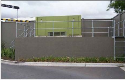
Figure 51 - Example substation raised above 1:100 flood level
