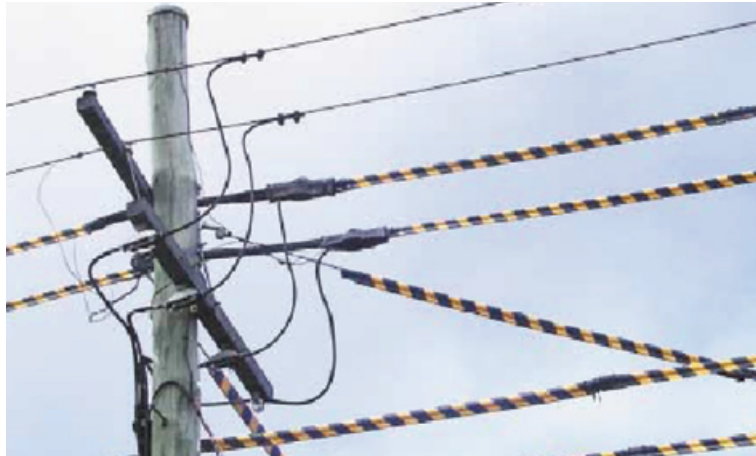
Figure 16 – Tiger tails fitted to overhead power lines
