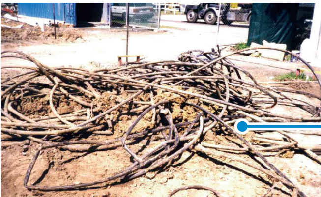
Sub-ducts and cables laying on the construction site, pulled out by an auger.
