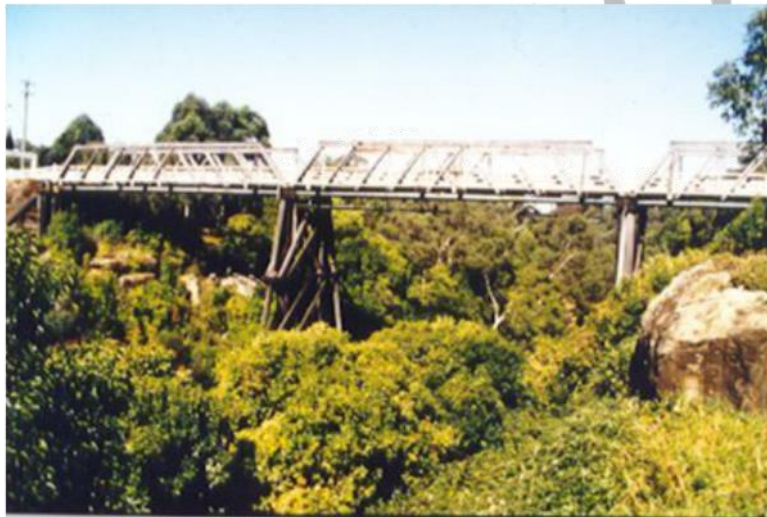
Figure 2: Constructed in 1897 Picton's Victoria Bridge, a timber truss bridge over Stonequarry Creek is still in use today
