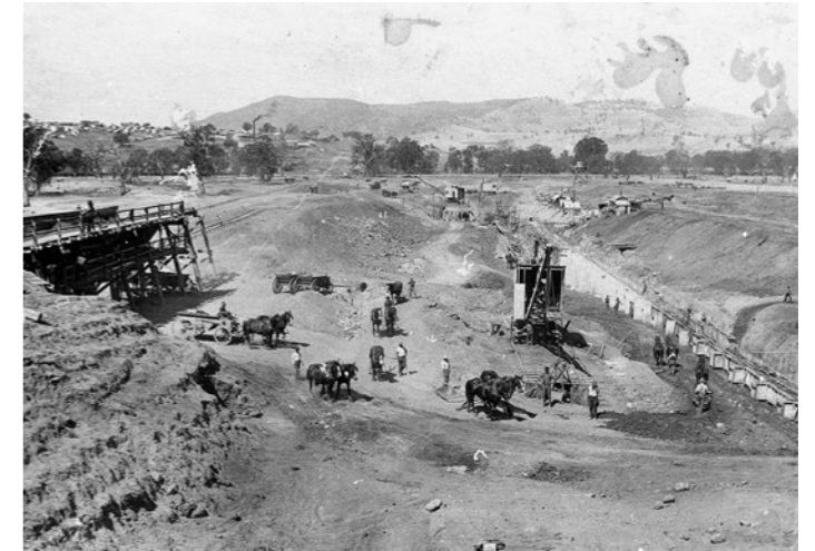
Figure 71. Hume Weir, 'Beginning construction of Hume Weir', Albury, 1920, accessed via the NSW State Library Archives
