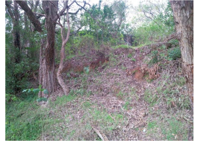
Fill embankment to the north of the access track, looking north toward the Norma Parker Centre wall at rear.
