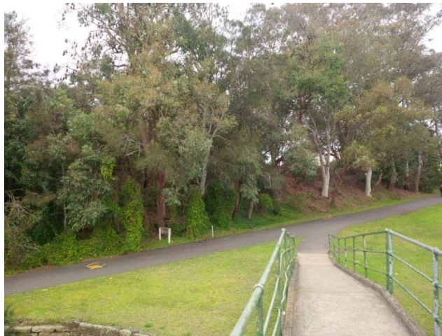
Scale of the fill embankment at the north-west site extent, looking toward Norma Parker Centre.
