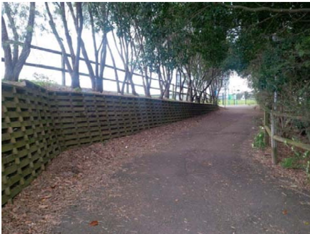
The access ramp from the practice field to the aquatic centre carpark, showing retention of practice field fill materia..
