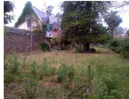
Norma Parker – Main Yard with fire damaged Building 108 on left (Pol AY)
