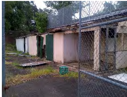
Norma Parker – Poor condition sheds (Building 110) (Pol 110)
