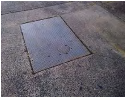
Linen Service - Suspected Heating Oil UST (Pol AE)
