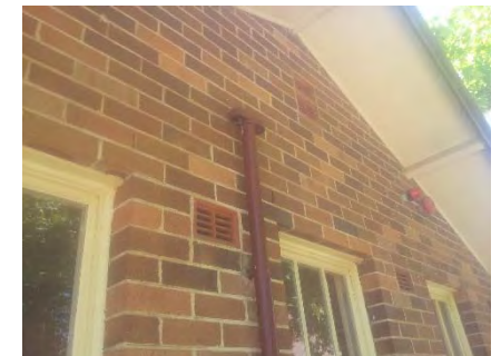
East Campus: Vent pipe on south wall of Building 54 (Pol AN)
