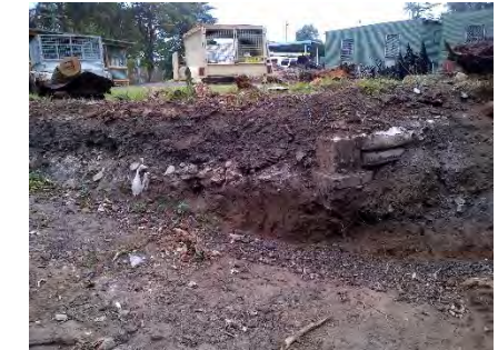
Vacant lands – Exposed cut face in fill material to north of Building 29, leading to access track to river bank.
