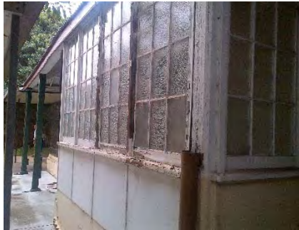
Norma Parker – Poor condition paint works and suspected ACM cladding at rear of Building 105.
