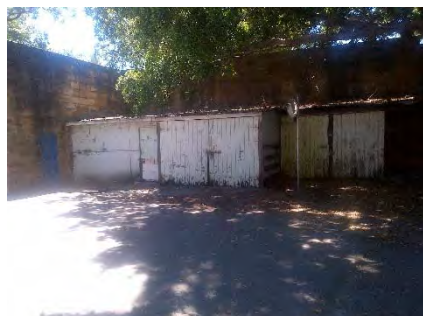
Building 91 – sheets, including ACM debris.
