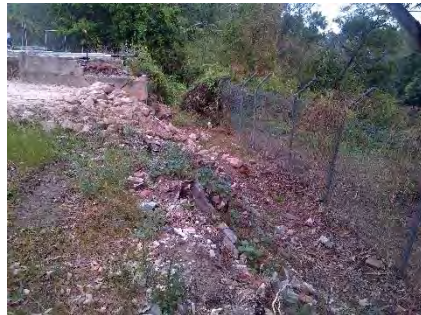
Vacant lands – South-west extent of SES Compound. Filled embankment with suspected ACM fragments exposed. (Pol AK)
