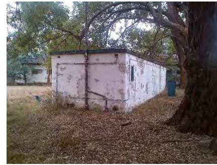
Vacant Lands – Building 10 air raid shelter with poor condition Paint work, looking toward the north-east, with Building 5 in background
