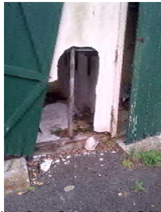
Norma Parker – Poor condition sheds (Building 110) (Pol 110)
