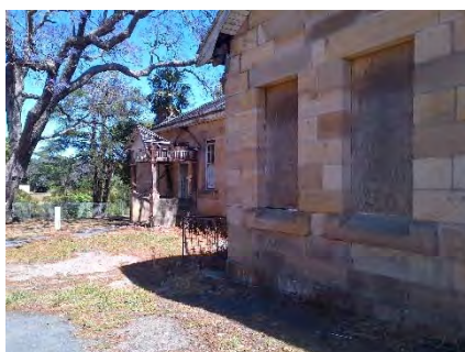
Fire Damaged Portion of Building 83
