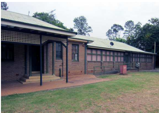
46 The Hospital Wing constructed in 1936 as part of the Girl's Industrial School.
