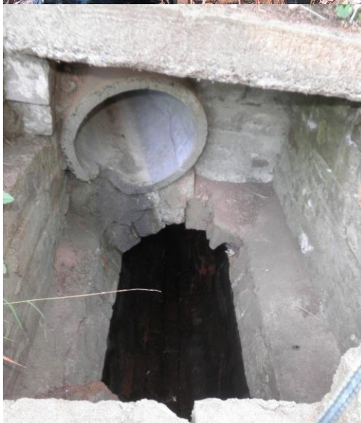
Figure 3.20: Detail showing break in drain and additional inlet. Note the construction of the main drain from bricks laid lengthwise (stretcher). Taken looking northeast, 29/07/2014, by NP.
