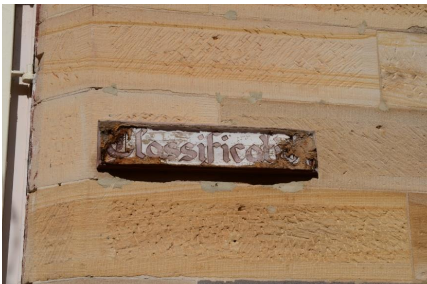
Figure 3.27: Detail of sandstone blocks on exterior of Wing 1 that appear to have been refaced. Photo taken 29/07/2014, by TL.
