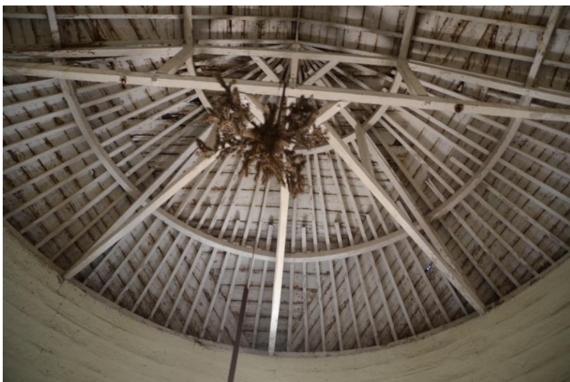
Figure 3.28: Timber ceiling in rounded, southeastern end of Wing 1. Photo taken 29/07/2014, by TL.
